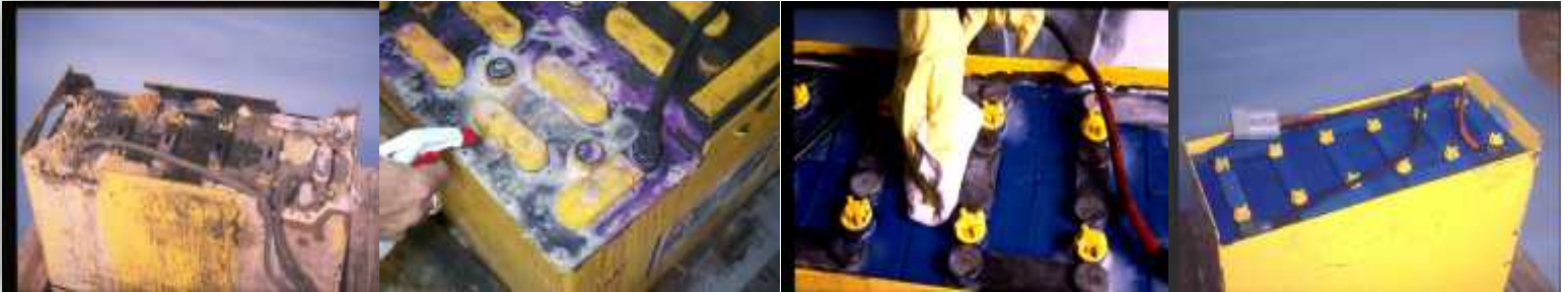
Fig.1 An example of a poorly maintained battery. This battery will require more charge time and, as a result, less work time.
